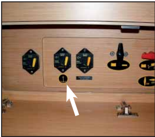
AUTOMATIC BREAKER OF THE WINDLASS
