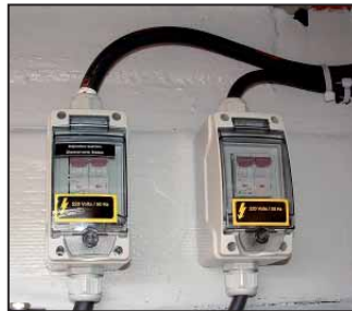
AUTOMATIC BREAKERS OF THE SHORE POWER SOCKETS
