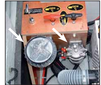
WATER FILTER + FUEL FILTER OF THE GENERATOR
