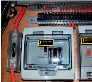
CONSUMING APPLIANCES CIRCUIT BREAKERS
