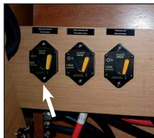
DAVITS CIRCUIT BREAKER
