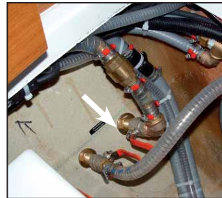
WATER INLET VALVE OF THE GENERATOR
