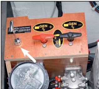
TANK / GENERATOR SELECTION PULL ROD
